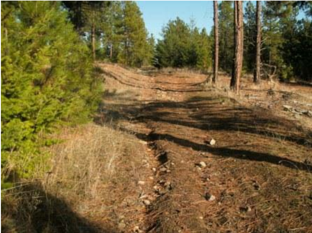
Photo 2: Minor rill erosion on existing unimproved road, east side of proposed project facility location.
